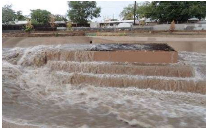
In-stream filtering structure at work during a June 2013 storm
